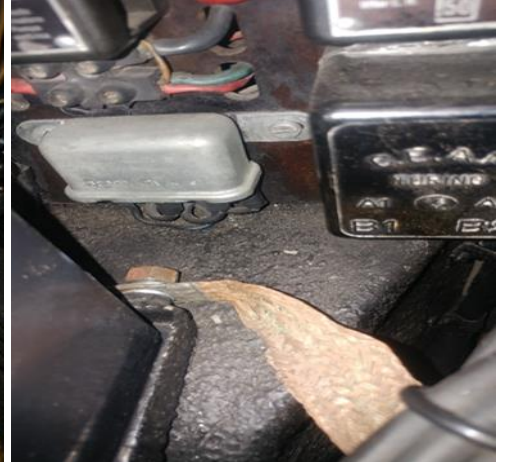
18) Copper ground strap
